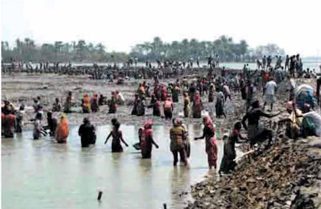
Local people repairing a damaged embankment after AILA in Munshiganj Union, Saikira district.
